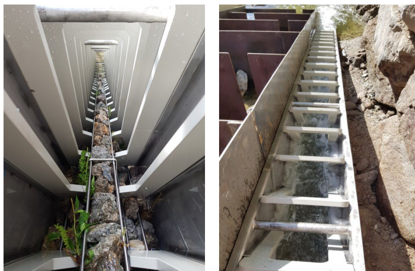
Figure 4. (Left): baffle geometry and substrate gabion. (Right): modified Denil fishway (MDF) in operation.
